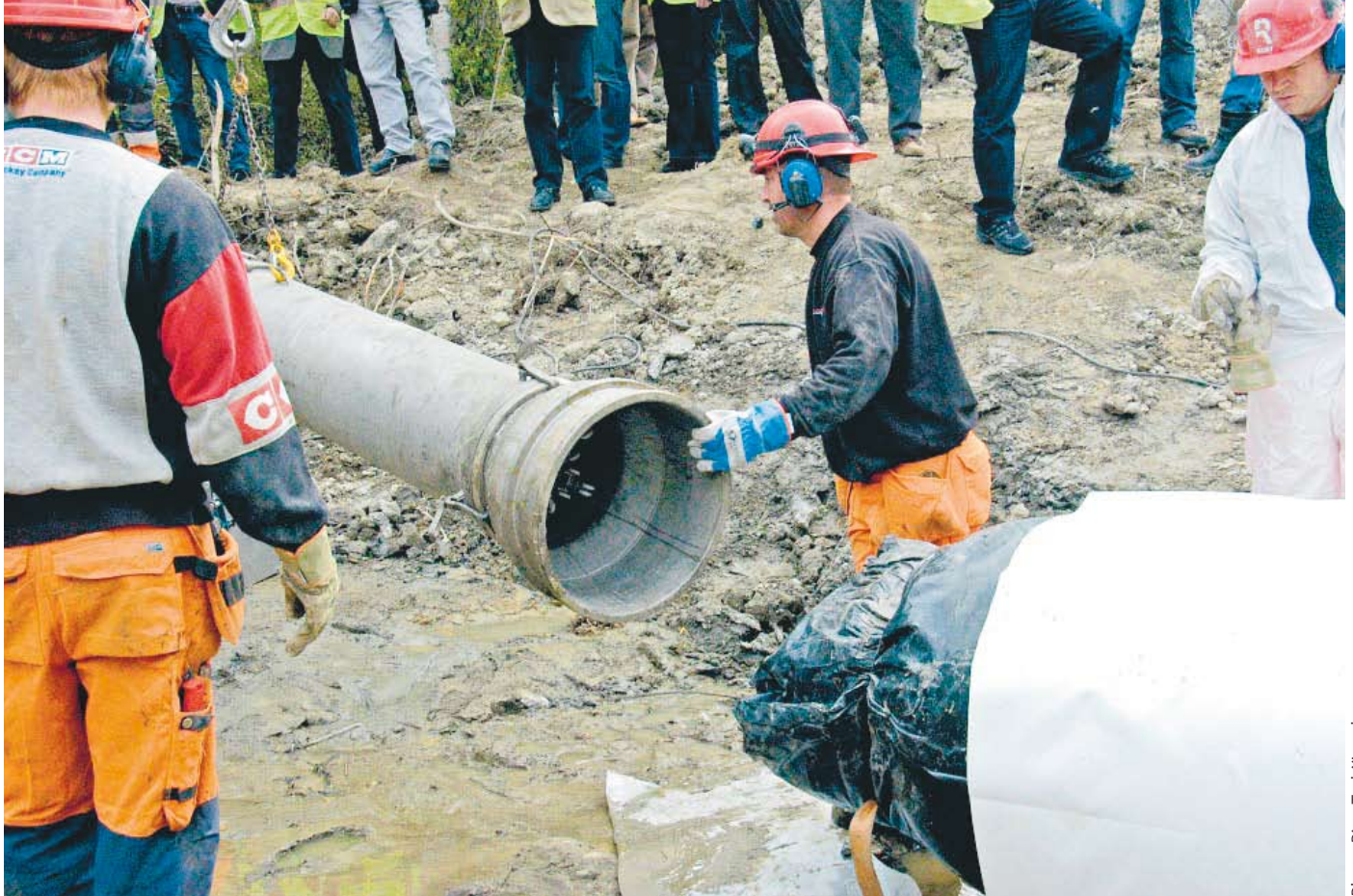
It is time for the Railcare team to remove the UV carriage pipe and the compressed air hose from the pipe liner. All that remains is to cut the excess fibreglass liner and receiving hose.
