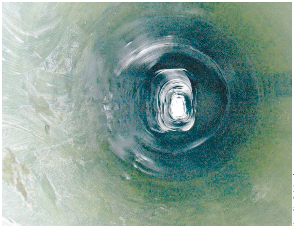
The fibreglass liner is perfectly flush with the culvert wall and is perfectly shaped to the square bit in the middle and the rounded ends.
